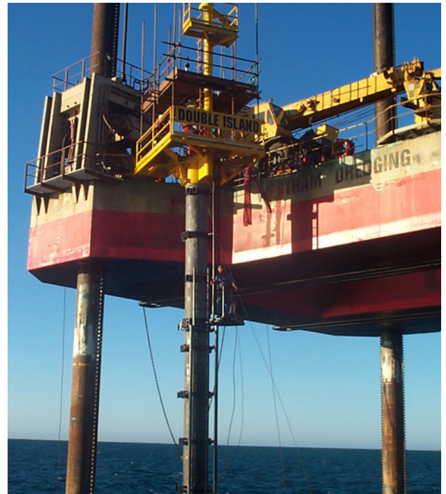
The "Sirius" self elevating platform located alongside the Double Island platform during installation
