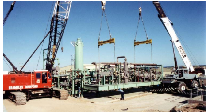
The gas plant was modular and skid mounted to minimise the installation time and cost.
