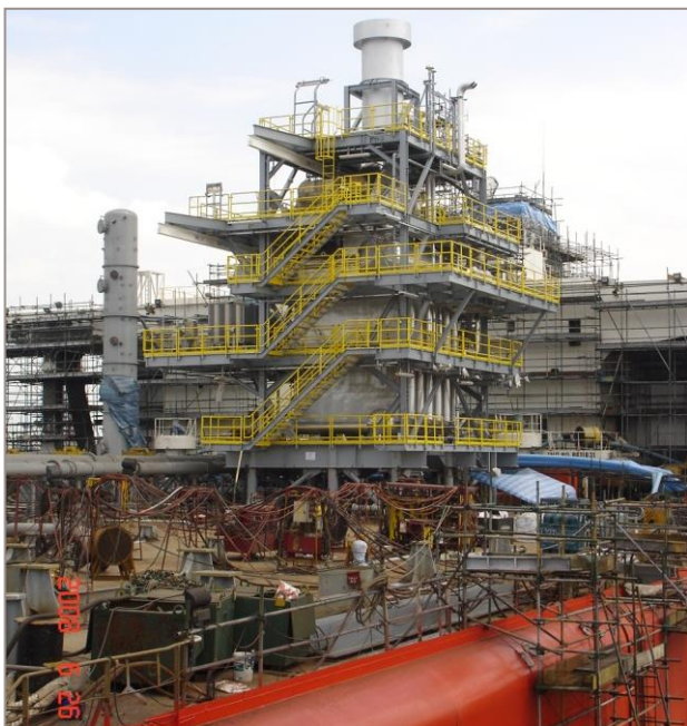
Aalborg boiler module installed on Azurite FDPSO
