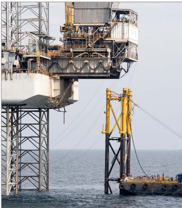
Jacket hung off aft end of barge and being upended at site
