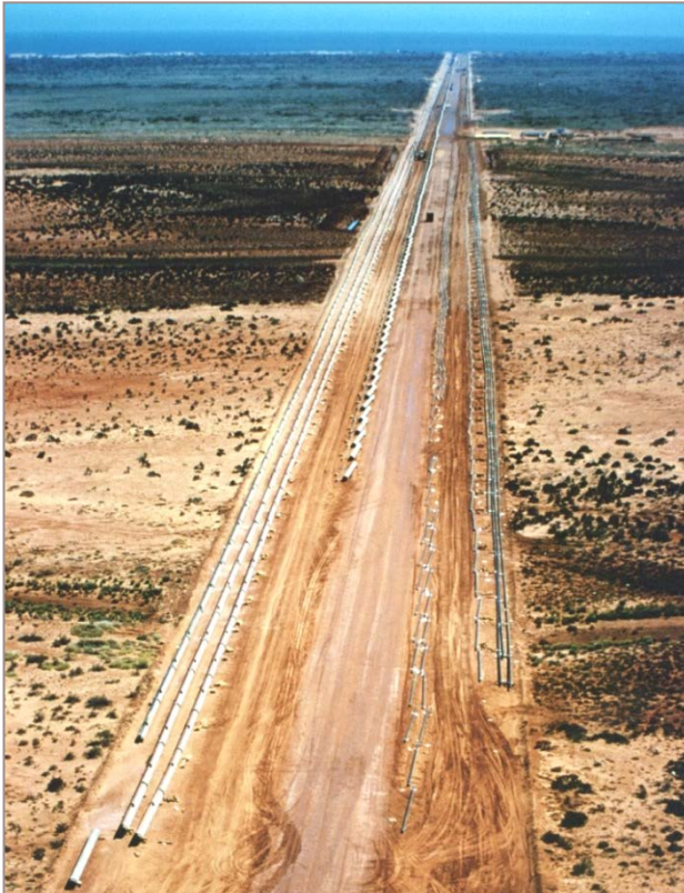
View of the pipeline string site at Tubridgi where the pipeline strings were made up prior to towing to site
