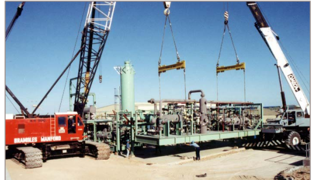
The gas plant was modular and skid mounted to minimise the installation time and cost
