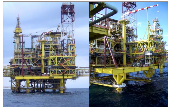
BRA Annexe installed with first process module in place
