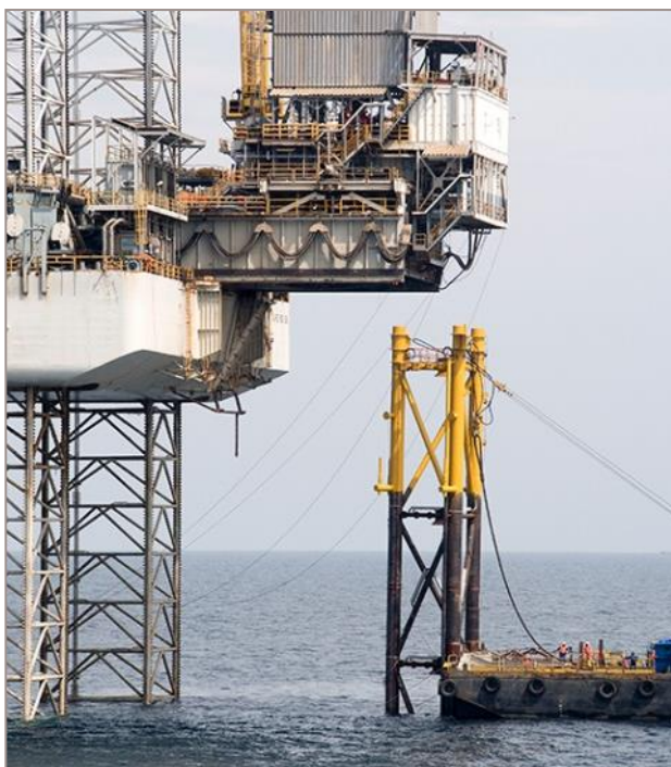
Jacket hung off the aft end of barge and being upended at site
