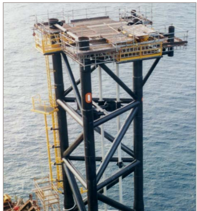
The upper substructure was transported vertically attached to the stern of the barge
